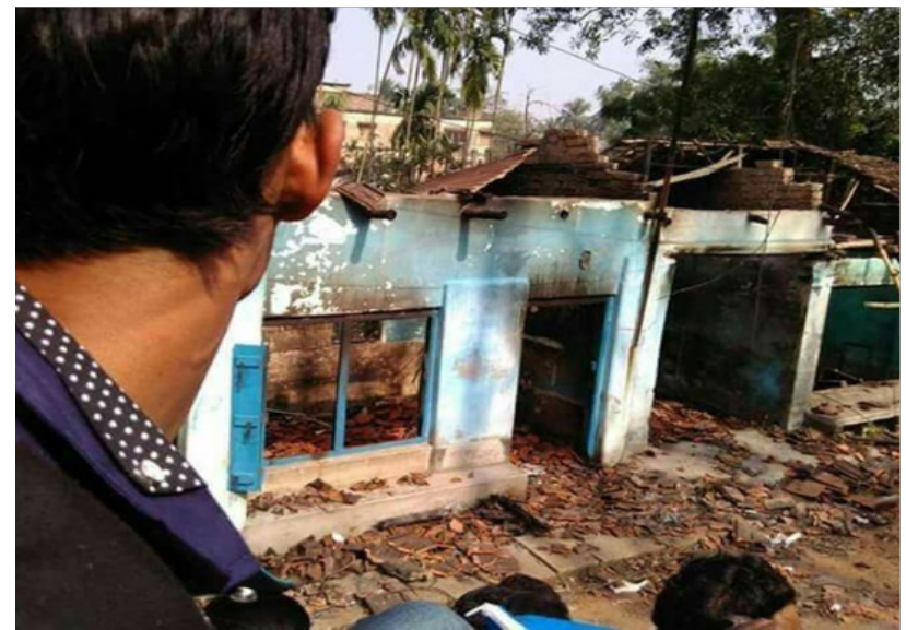
Burnt House in Katwa Riots
